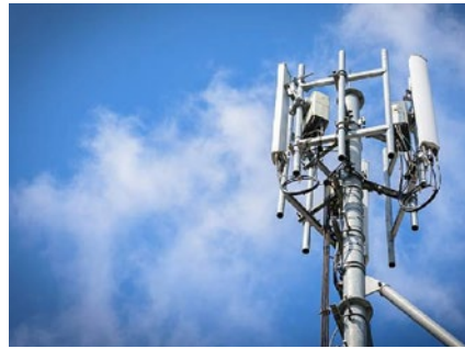
MOBILE BASE STATION
