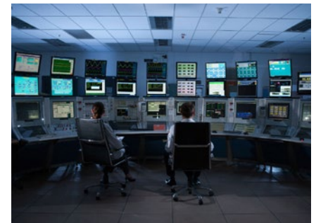
VIDEO SURVEILLANCE ROOM
